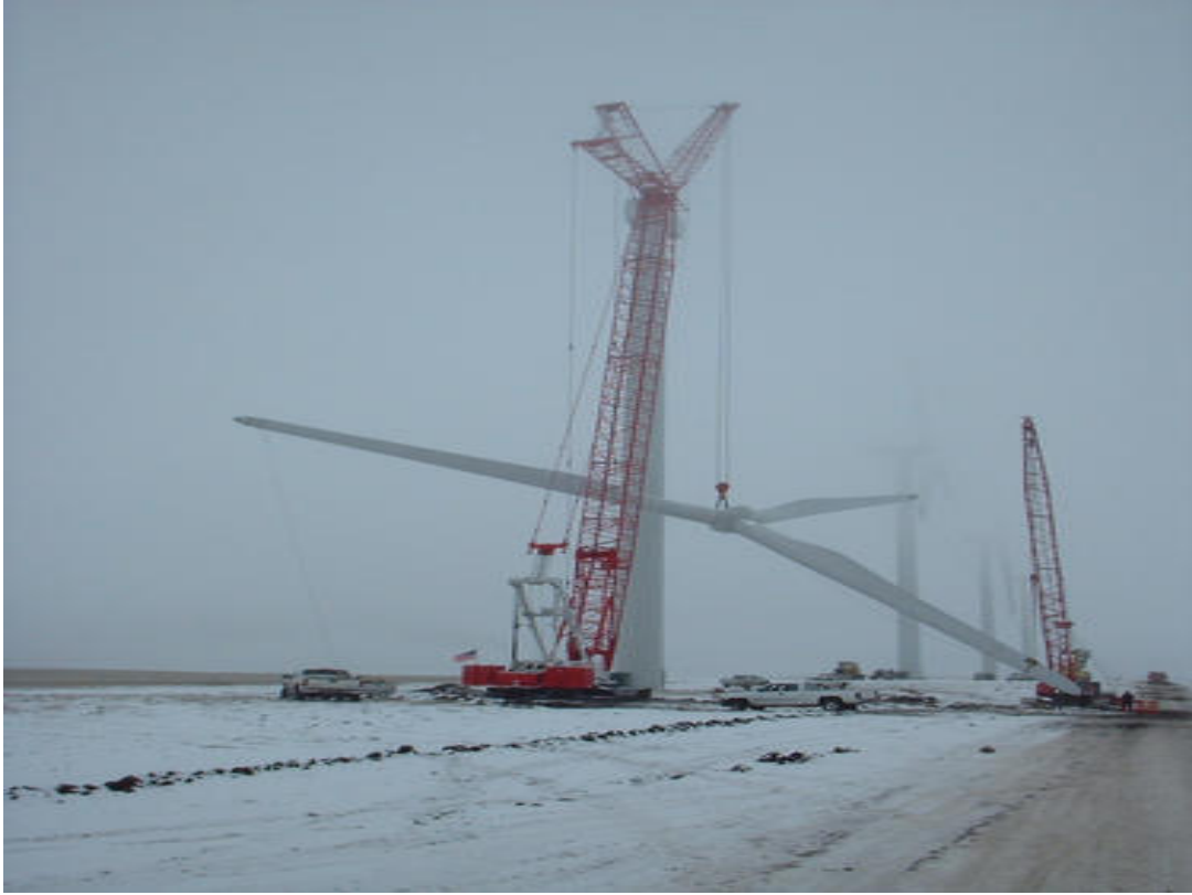
FIGURE 3.1.2-3 Installation of a Rotor on a General Electric 1.5-MW Wind Turbine at the Klondike, Oregon, Wind Farm (Source: NREL 2004c, Photo #11919. Photo credit: Paul Woodin.)
