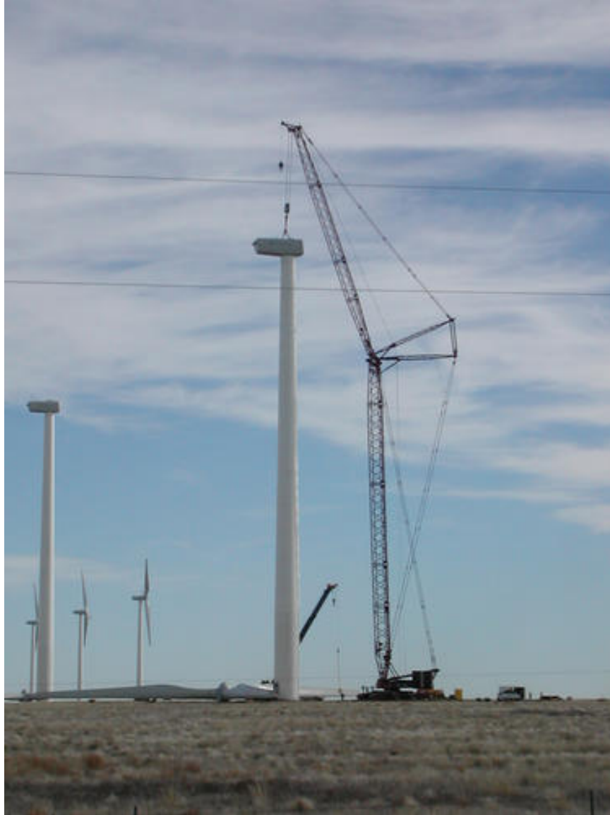
FIGURE 3.1.2-2 Wind Turbine Nacelle Installation at Golden Prairie Wind Farm, Lamar, Colorado (Source: NREL 2004b. Photo # 13060. Photo credit: David Jager.)
