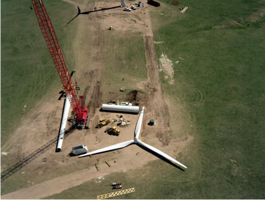
FIGURE 3.1.2-1 Aerial View of Preparations to Erect a Wind Turbine Tower at the Public Service of Colorado Ponnequin Wind Farm, Weld County, Colorado (Source: NREL 2004a, Photo #08607. Photo credit: Warren Getz.)
